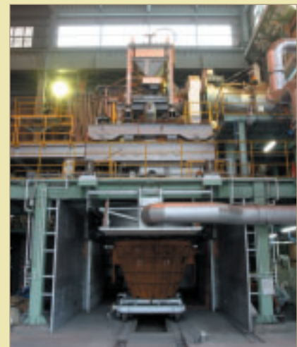
A DSR furnace
